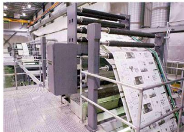
At Transcontinental Metropolitan, a Goss Mainstream 80 was erected in a new plant built to produce the French-language
